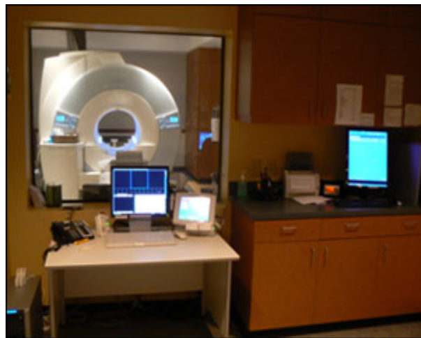
Photo by Mark A. Brown The typical MRI unit set up in a medical facility.
